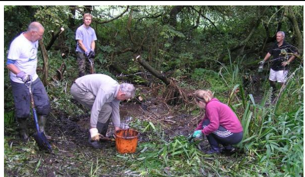
Clearing one of the ponds in the carr at Moorend Spout. (A carr is a wet woodland, usually with willow and alder). This pond is more like a swamp and it can be dangerous!
