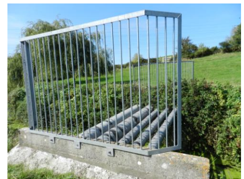
MoD kerosene pipes crossing the Land Yeo These pipes run the length of our field They have recently been refurbished at this point (see below- photo by Hilary West)
